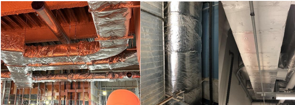
Flexible Wrap on Rectangular Duct
