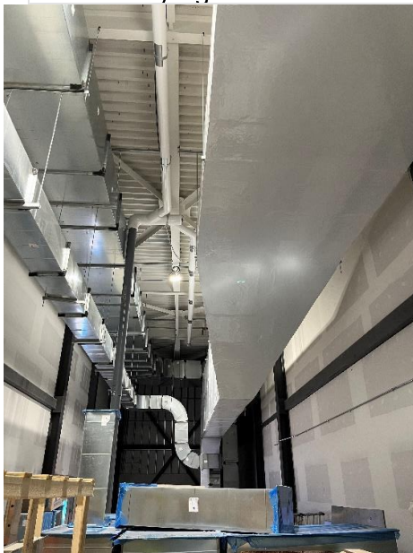
Duct supports outside of insulation envelope
